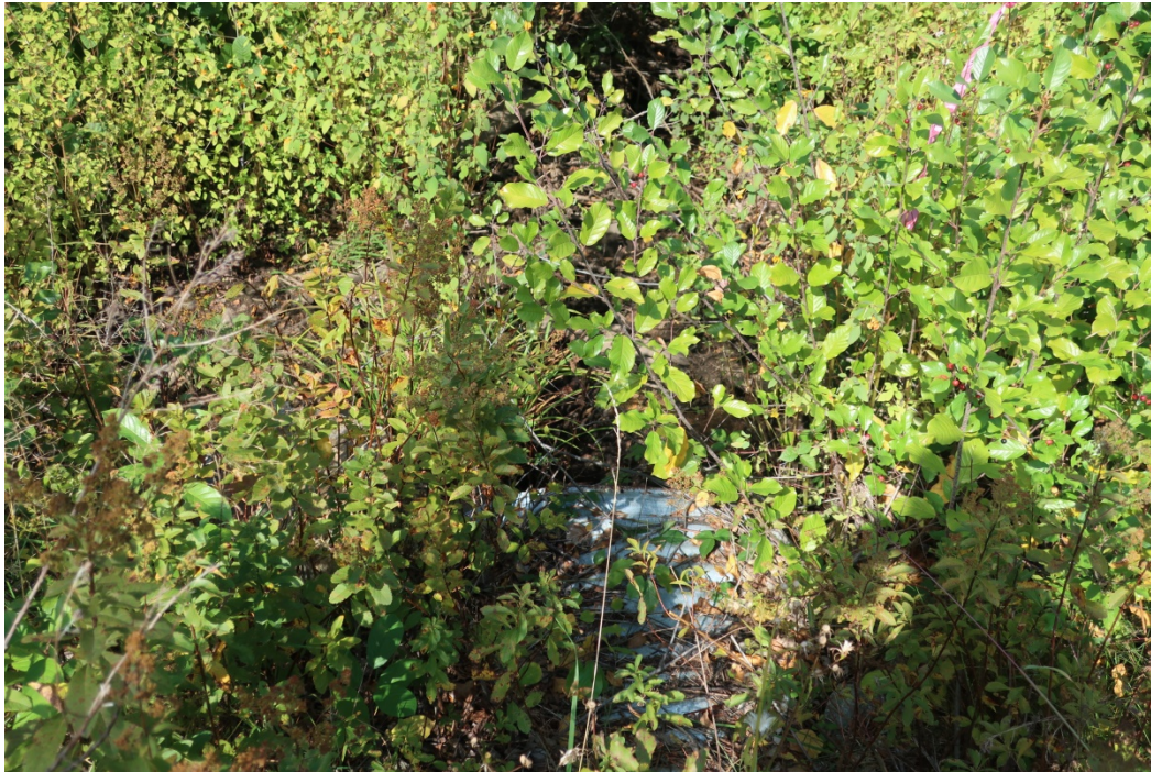
Culvert location, north side of Portland Street. Note dense shrub community Photo taken on September 30, 2019
