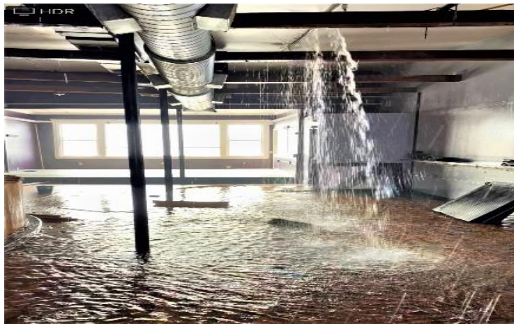
Froze and burst sprinkler pipes on North Main Street
